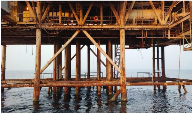
Figure 2. General Condition of Members in Splash zone
