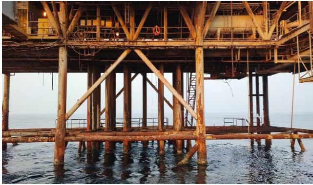
Figure 2. General Condition of Members in Splash zone
